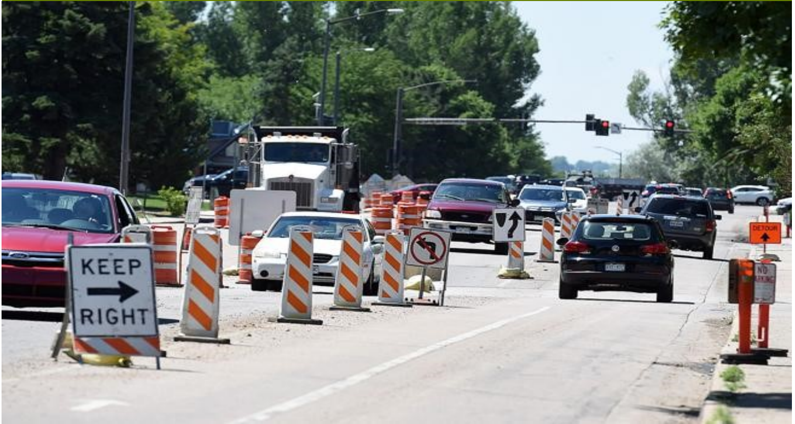
Cars maneuver through road construction zone on Boise Ave north of Eisenhower Blvd in Loveland. Image Credit: Jenny Sparks / Loveland Reporter-Herald
