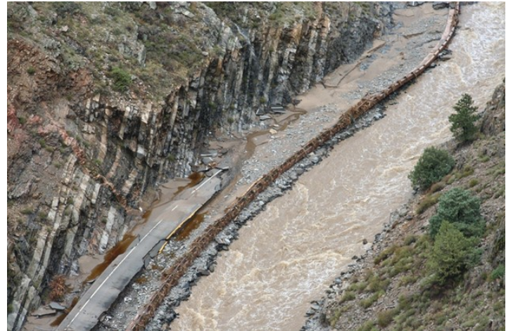
Damage to US 34 from 2013 Floods Image Credit: CDOT
