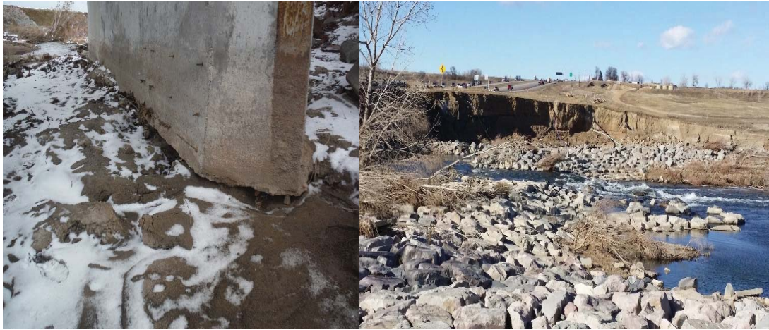
Scour Damage at the Big Thompson River and St. Vrain Creek
