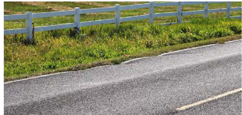
County roads experience deterioration at a faster rate when traffic volumes increase: Rutting in wheel tracks and poor shoulder conditions are evident in this view of Weld County Road 23 north of Severance.
