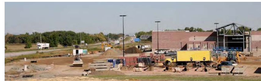
Looking north from Harmony Road at Interstate 25 (left) and the Timnath Walmart Supercenter under construction in 2008 (right).
